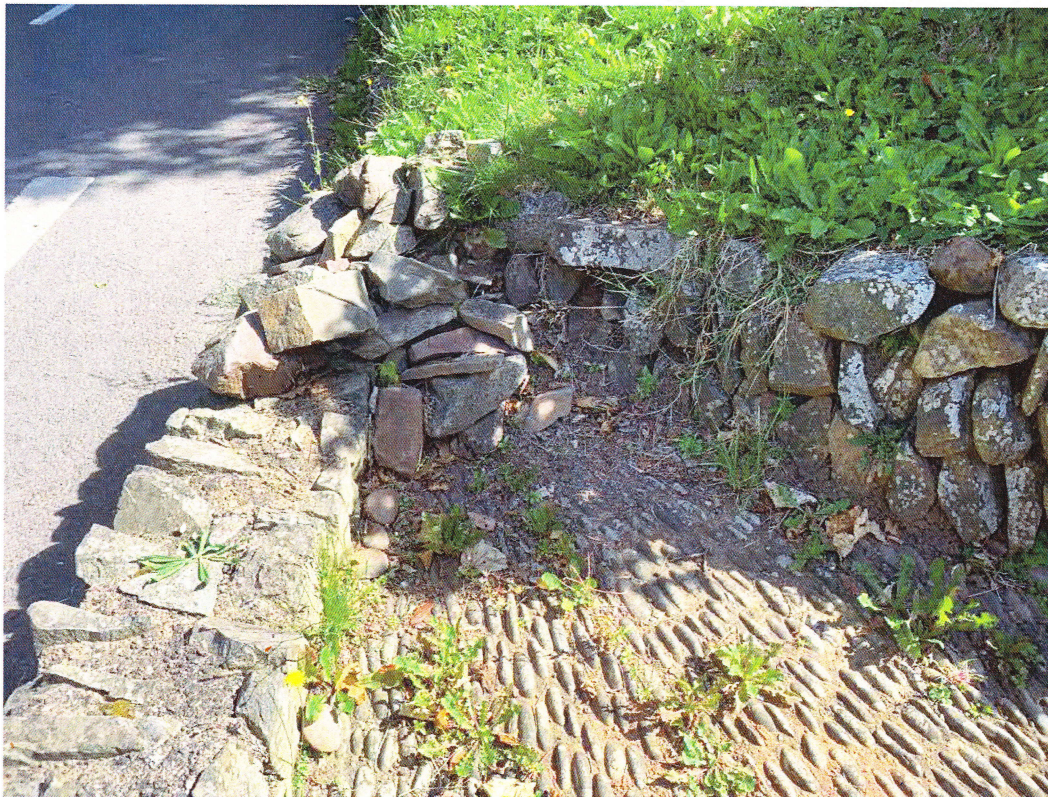
North-West corner of the walled area has suffered a partial collapse and requires re-building.
