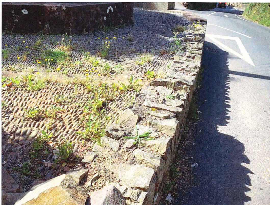
The remaining areas of walling require vegetation removal and re-pointing as necessary to prevent further deterioration.
